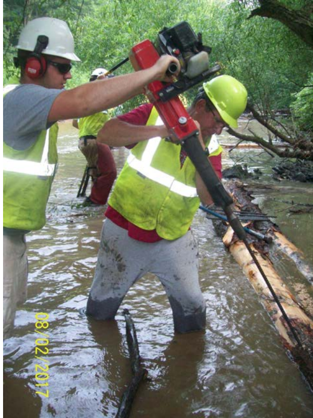
Unusual silt depth requires extra long 6 foot rods being used pinning logs into streambed.
