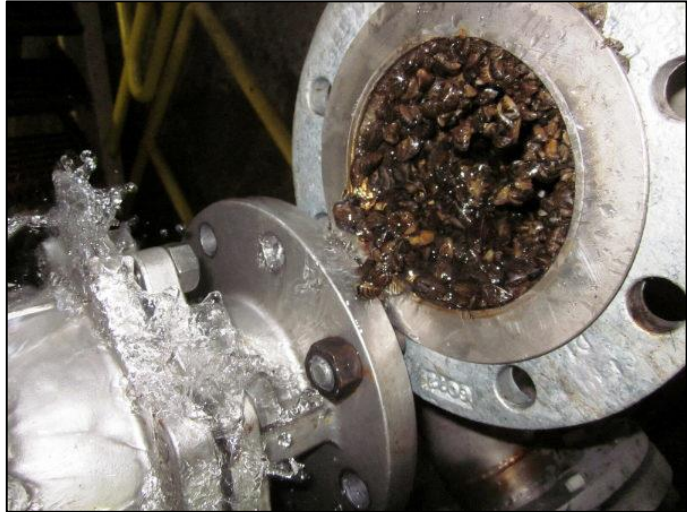
Photo 31. An example of zebra mussel cluster clogging a water intake pipe.
