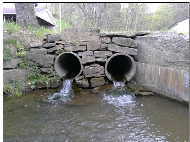
Photo 16. Example of stream crossing culvert allowing No AOP.
