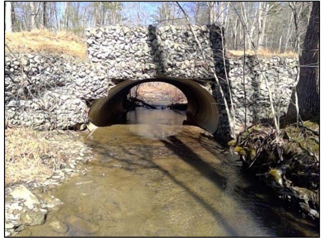
Photo 15. Example of stream crossing culvert allowing AOP.
