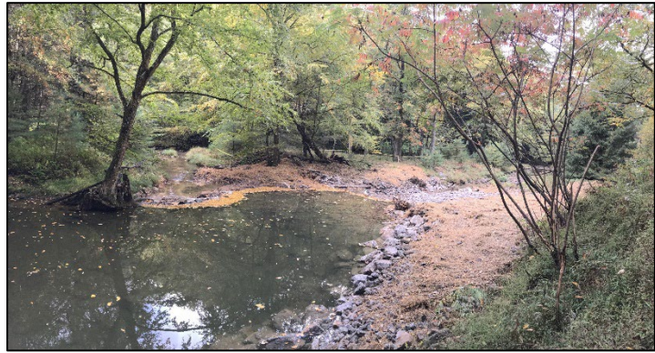
After work was completed on Phase I in 2020, a temporary grade control rock dam had to be constructed at the entrance to the side channel to maintain flow in both channels until additional construction could be completed on Phase II in 2021.
